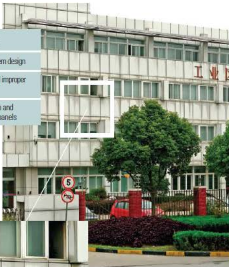
BUILDING CLEANED REGULARLY BUT STAINING CANNOT BE REMOVED
